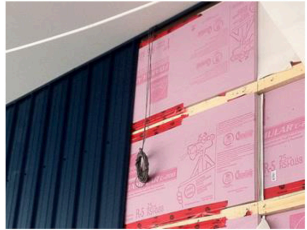
FIGURE 4 | The second layer of XPS is shown in place over 6 mm polyurethane foam. The XPS layer ensured that the bottom surface of each VIP was attached to a smooth surface and protected from abrasion. A layer of 6 mm flexible polyurethane foam was placed over the exterior surface of the VIPs to help prevent mechanical rubbing of the outside surface of each VIP against the 25 mm polystyrene foam board placed on top of it.
