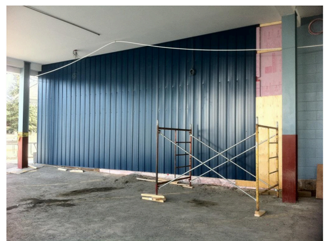
FIGURE 5 | Post-retrofit wall (MacLean and Korn, 2011). Because all holes for fasteners were drilled before the siding was put on the wall, it was possible to visually check that all fastening points were directly over the support members.
