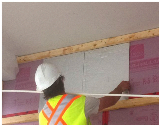
FIGURE 3 | Installation of VIPs over a layer of XPS and a 0.15 mm (6 mil) polyethylene air vapor barrier on the existing concrete block wall (MacLean and Korn, 2011).
