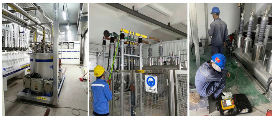
FIGURE 9 Integration and pre-commissioning field test.
