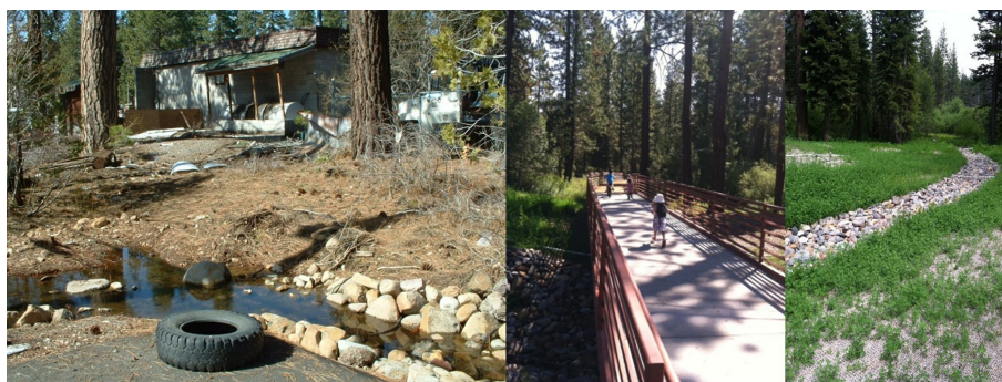
FIGURE 3 Snow Creek Wetlands restoration project before (left) and after (middle, right) cleanup. Photo credits: Kansas McGahan (left) and Placer County (middle, right).
