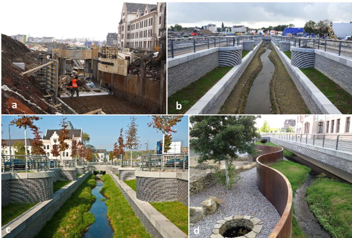
FIGURE 8 Hörder Bach restoration process including (a) preparation for the daylighting in front of Hölder castle, (b) daylighting Hölder stream via removal of part of the street. (c) Hölder stream a few years after daylighting. (d) Historical excavations and the lower section of Hölder stream in front of Hölder castle. Photograph: (a) Frank Schultze, (b) Jochen Durchleuchter, (c) Gabi Lyko, (d) Nadine Gerner, all Emschergenossenschaft.
