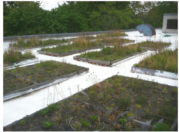
FIGURE 2 | Example of green roof plots installed on New York City Department of Parks and Recreation recreation center roofs in fall of 2010, consisting of 12 planter boxes measuring 4 m x 2 m, for a total area of 96 m 2 . Roofs were surveyed for bird activity and bird species richness in May of 2010, 2011, 2012, and 2014.
