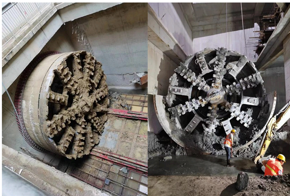
FIGURE 12 Abrasion diagram of the cutter after the shield crosses the anchor cable zone.
