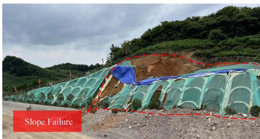
FIGURE 9 The on-site real image of the final slope collapse.
