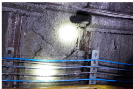
(a) Roof peeling
