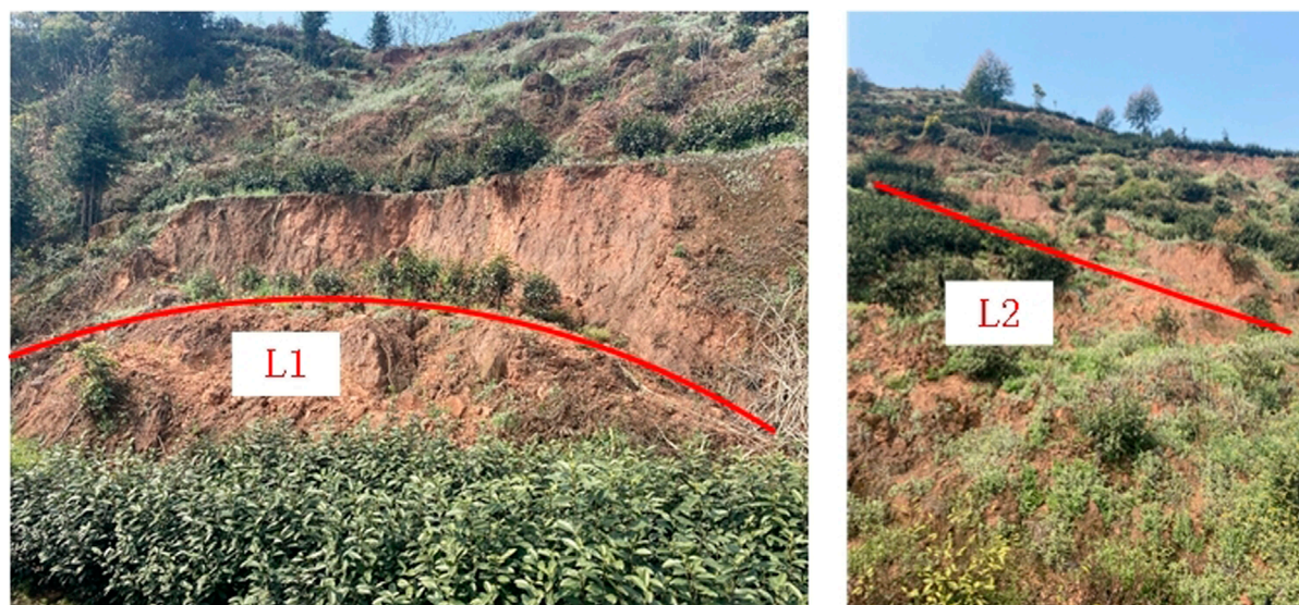
FIGURE 1 Local landslide cracks.
