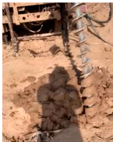
(b) Saturated loess in a deep displacement borehole
