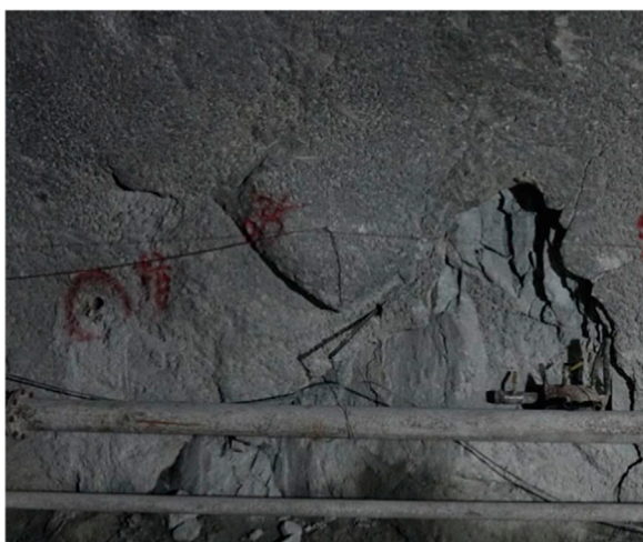
FIGURE 16 Cracking area of the DK199+655~605 section of the entrance tunnel.
