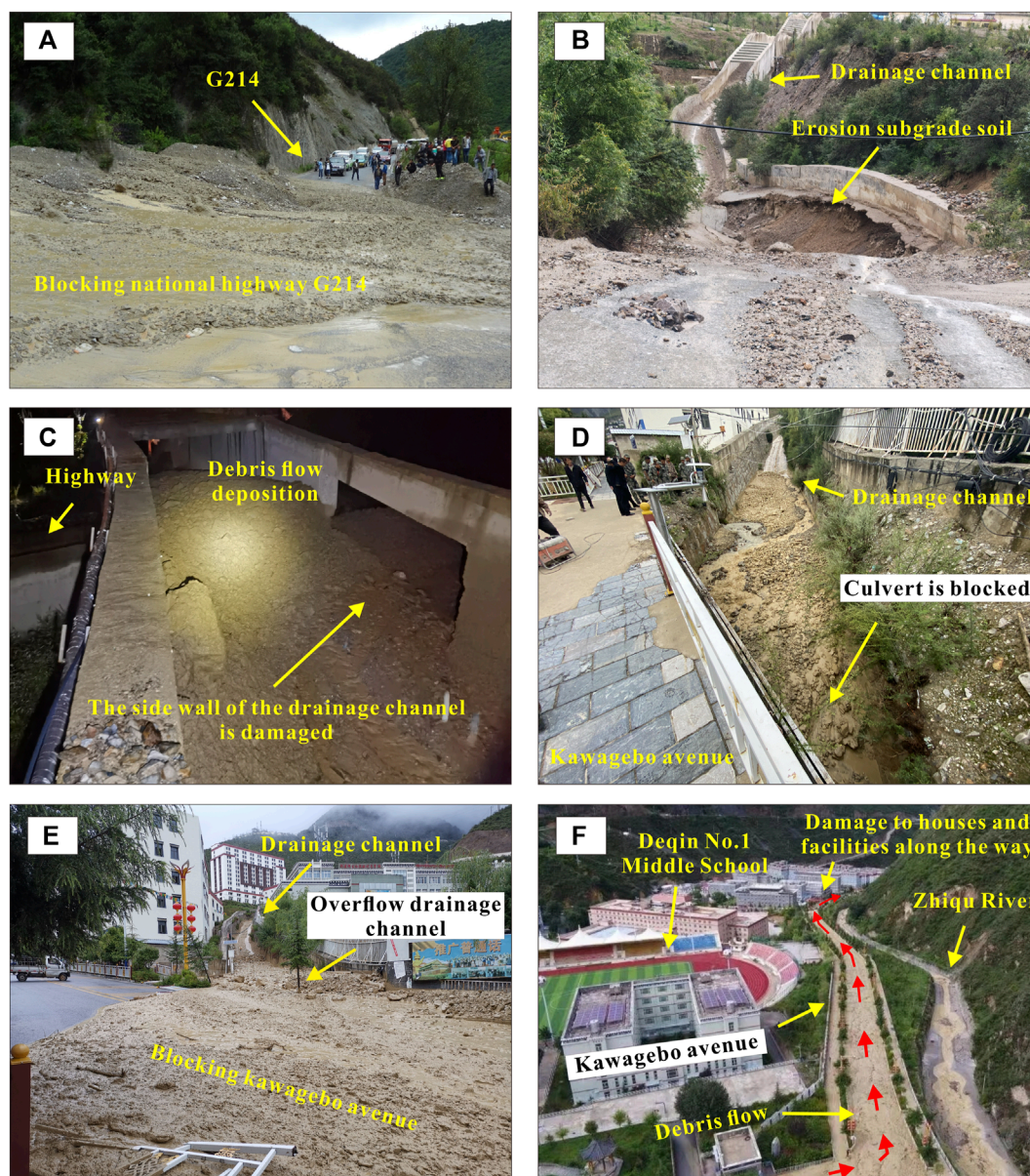
FIGURE 9 Debris flow outbreak situation. (A) blockage of national highway G214; (B) erosion of the drainage channel; (C) damage to the side walls of the drainage channel causing debris flow spillage; (D) blockage of the culvert; (E) Debris flow overflowing the culvert; (F) Debris flowing down the Kawagebo avenue.
