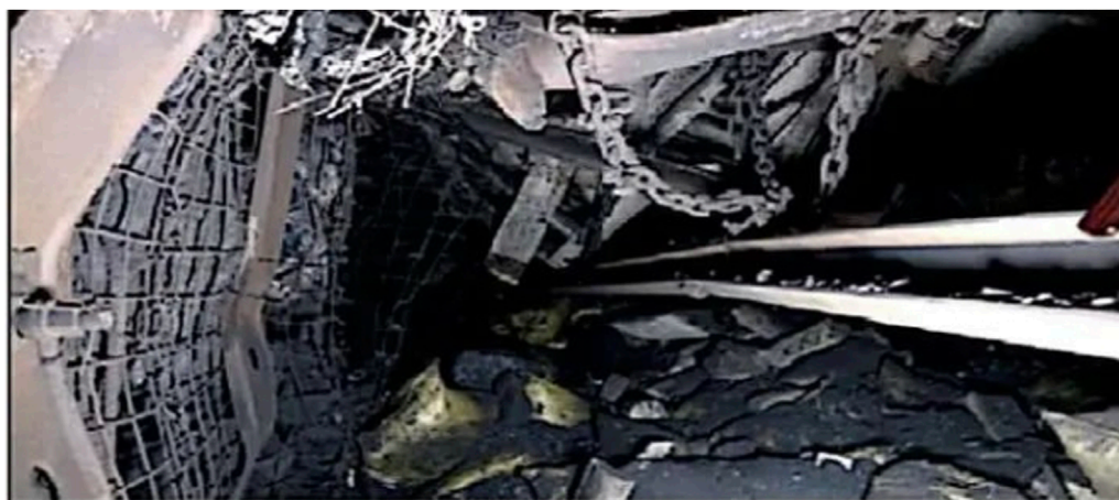
FIGURE 1 Damage situation of the roadway at Longgu Mine from 24 m to 40 m on the upper entrance of Sanlian Tunnel.
