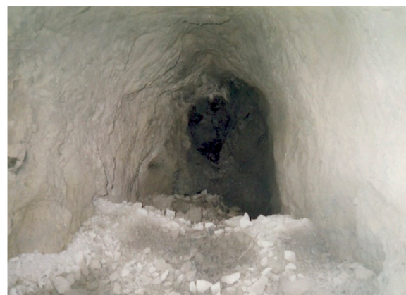
FIGURE 3 State of the bottomhole within the Belousovski field after blasting the snubber blastholes of the first and second sections.
