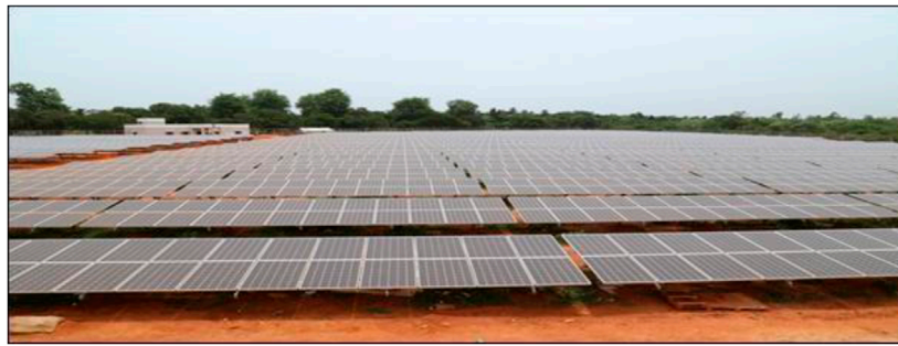
FIGURE 9 Solar power panels at Block-4, Neyveli, Neyveli Lignite Corporation, Ltd., India.
