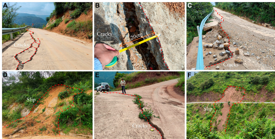
FIGURE 10 Photographs of LuJiaZhai–DaPingDi Minefield survey: (D) and (F) depict pronounced sliding on steep slopes under bush cover; (A), (B), (C) and (E) illustrate road damage caused by subsidence.
