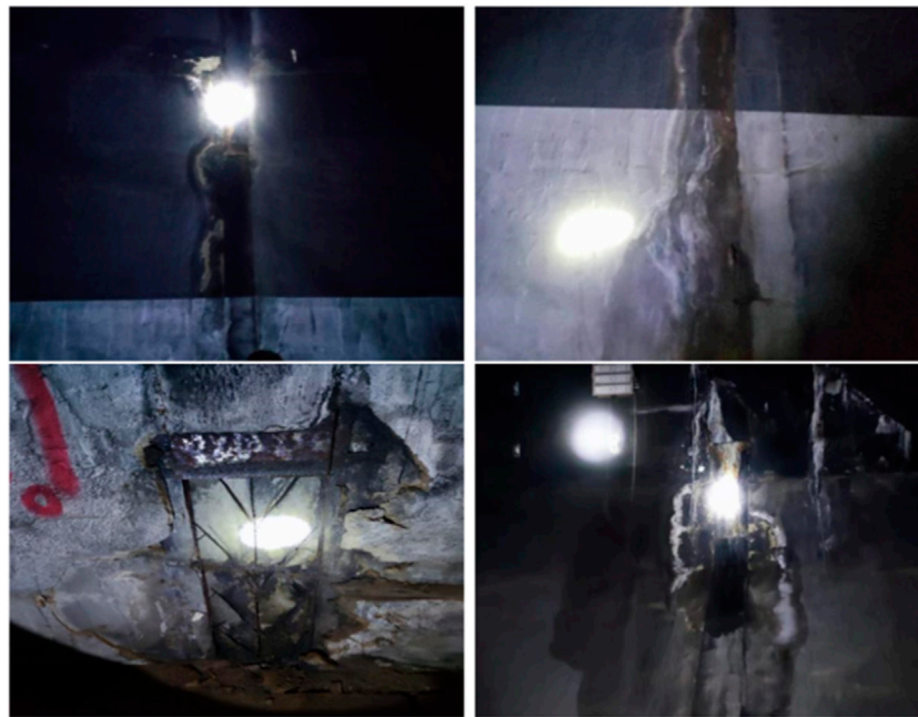
FIGURE 8 The image of water leakage disease in Huangmeishan Tunnel.
