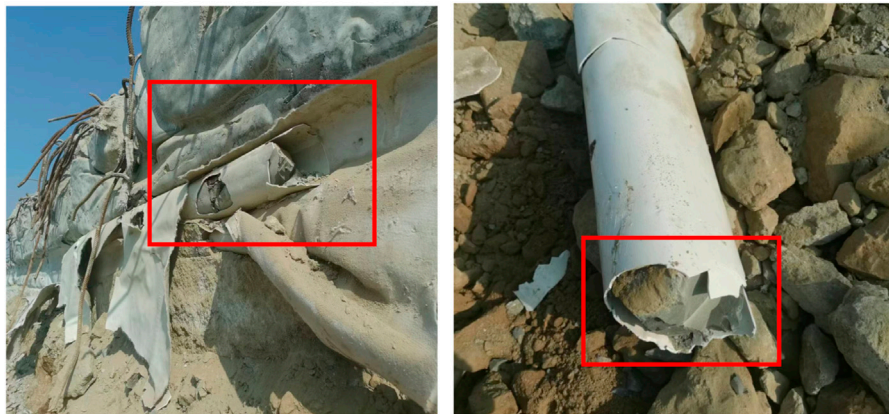
FIGURE 11 The clogged drainpipe in the Huangmeishan Tunnel.
