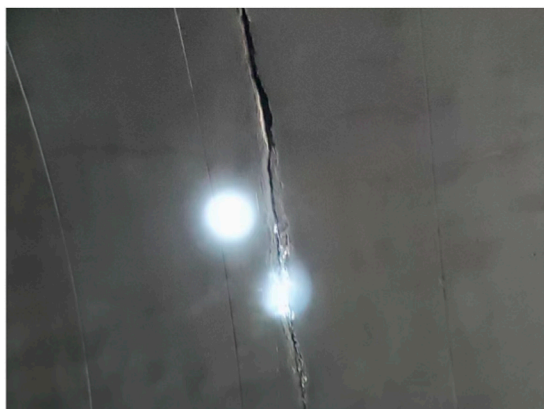
FIGURE 15 Crack at section YK4+576.
