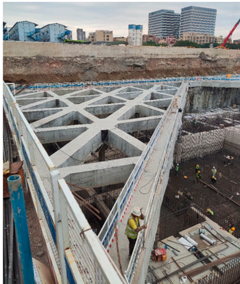
FIGURE 7 Site photo of the ground connection wall of the transfer channel foundation pit after general excavation.
