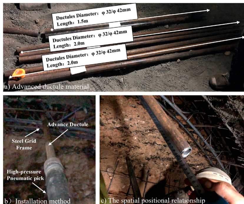
FIGURE 3 Schematic diagram of using small conduits and installation methods in the experiment.
