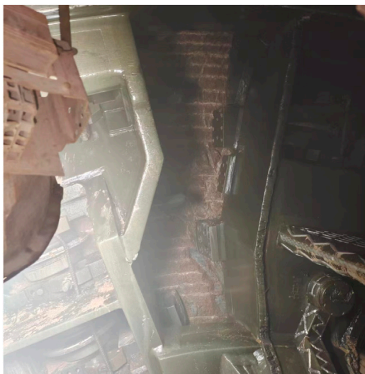
FIGURE 8 Tunnel surface of the 205th ring in the Shanwu tunnel section.
