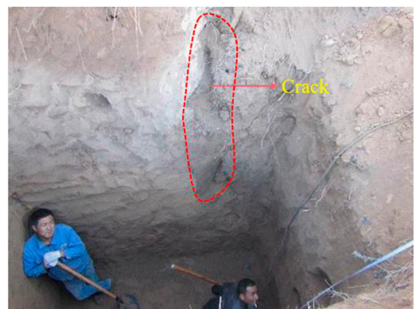
FIGURE 6 H1-2 east boundary shear crack (SK1).
