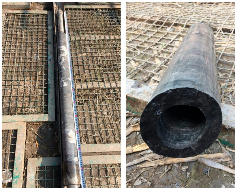
FIGURE 7 Photos of site application (the device and ring core are successfully recovered from the borehole).
