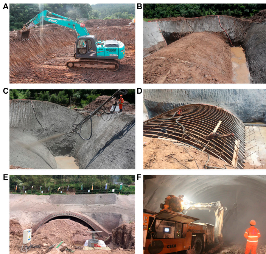
FIGURE 15 Site construction diagram of shallow-buried cover excavation section I: (A) Slope excavation and dressing; (B) Schematic diagram of soil mold; (C) Soil arch hardening treatment; (D) I-beam installation and split screw installation; (E) Excavation of underground tunnel; (F) Initial shotcrete support.
