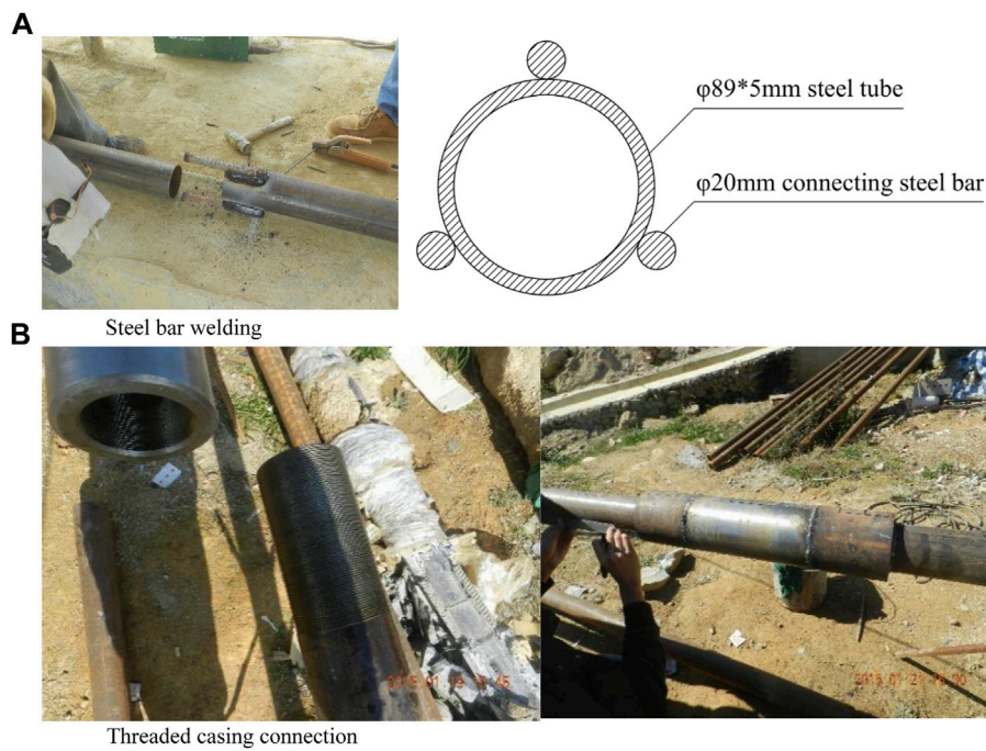
FIGURE 1 Steel bar welding and threaded casing connection. (A) Steel bar welding. (B) Threaded casing connection.
