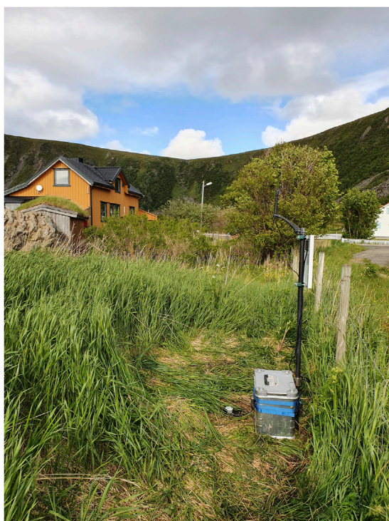
FIGURE 7 Environmental monitoring station installed at the settlement mound Sjøberget, Andøya. Note the solar panels on top of the logger cabinet. Photo: Vibeke Vandrup Martens, NIKU 2021.
