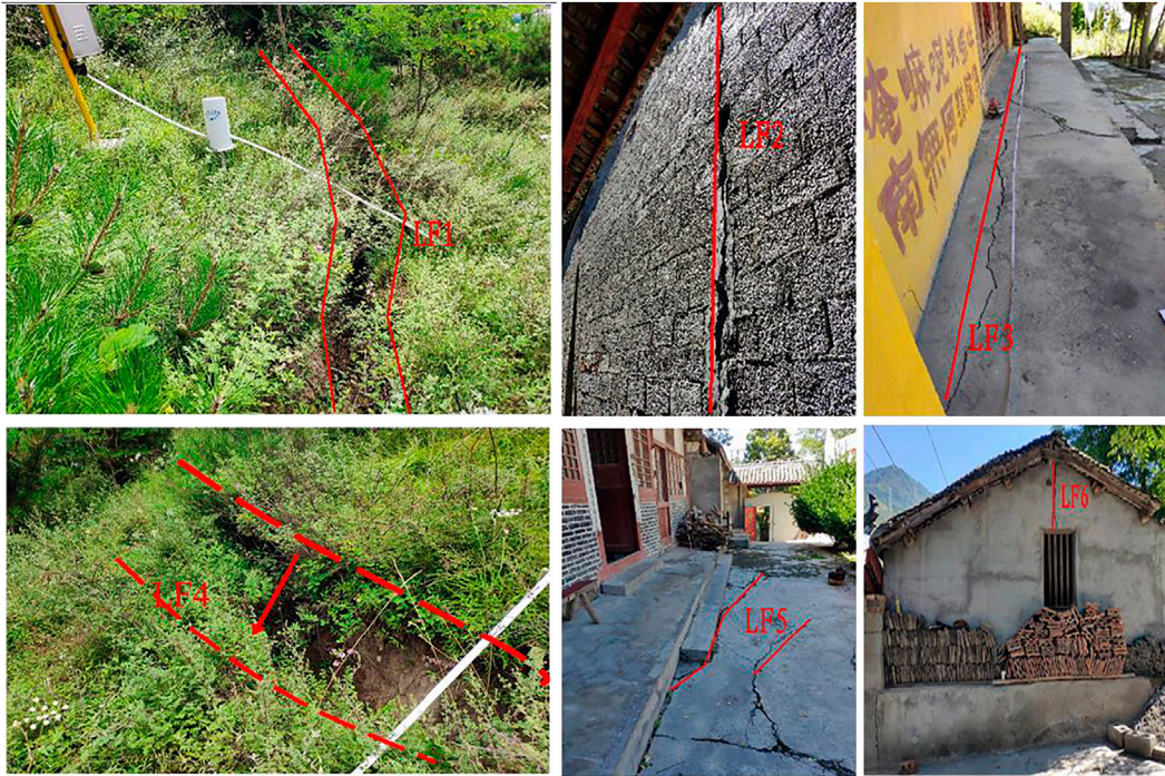
FIGURE 1 | Cracks measured by the GPS points on the front part of the slope.
