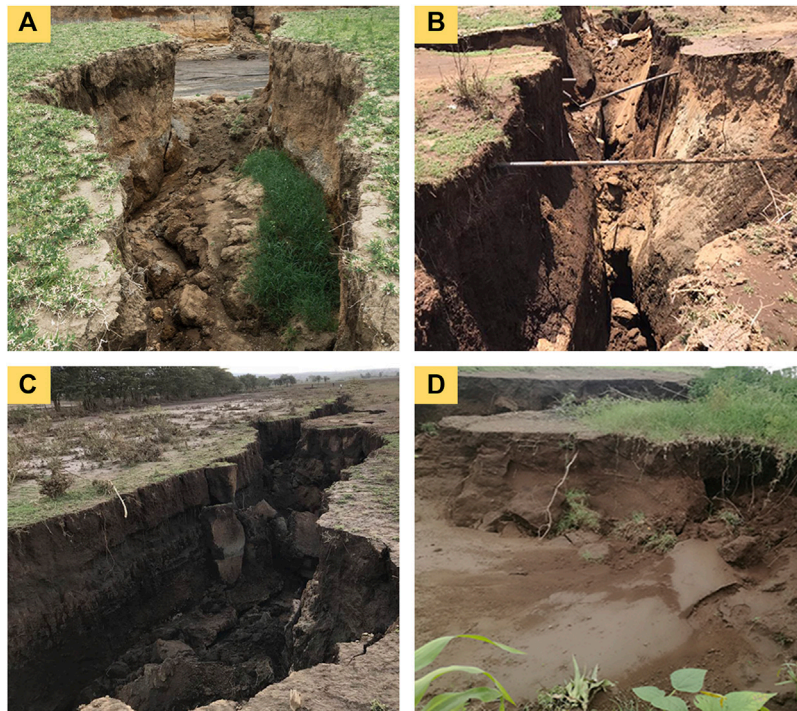
FIGURE 2 | Scene photos of ground fissures near the railway. (A) DK76; (B) B3 highway; (C) DK77; (D) ground fissure through a pond.
