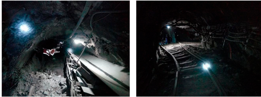
FIGURE 9 | Field investigation on the deformation status of the 11 coal belt roadway.
