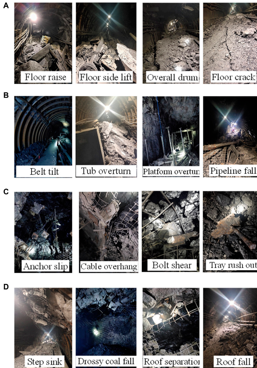
FIGURE 5 | Pictures of burst failure of coal burst on site. (A) Floor bulge; (B) Equipment damage; (C) Support failure; (D) Roof caving.
