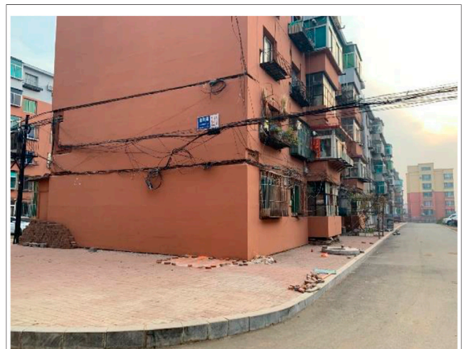
FIGURE 8 | Separation of building a wall from the foundation in feature-3 area.
