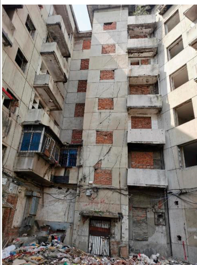
FIGURE 7 | Cracking of building wall and damage of balcony in feature-2 area.
