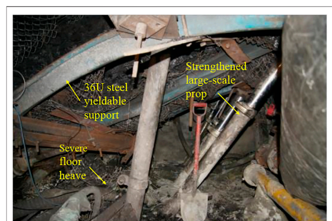
FIGURE 4 | Site photograph of rockburst in the head entry of the 21,221 working face.
