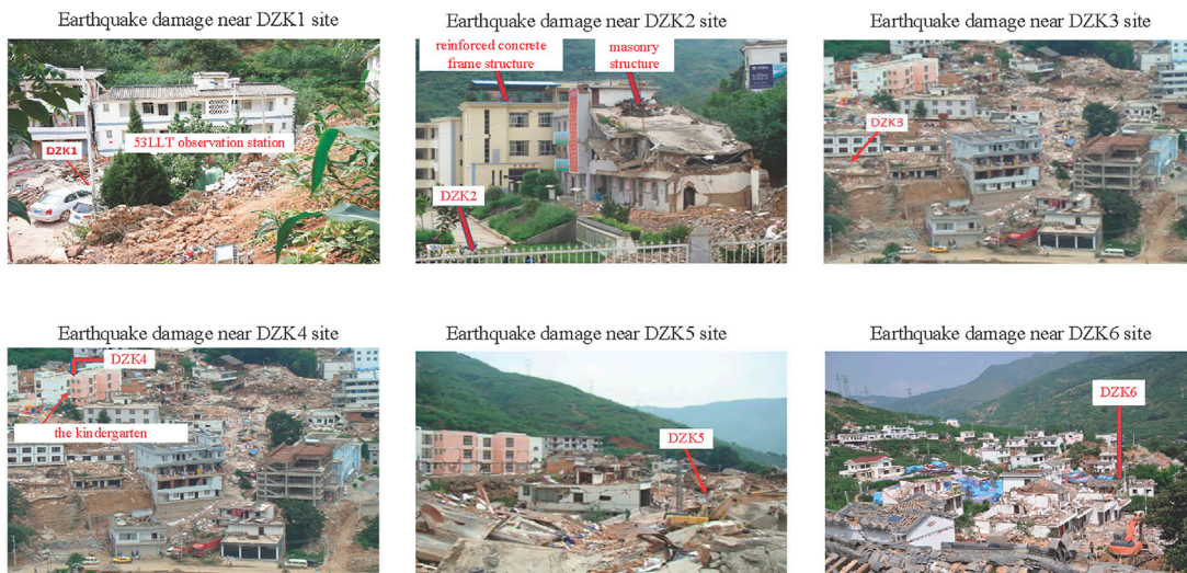
FIGURE 8 Earthquake damage in Longtoushan Market Town.
