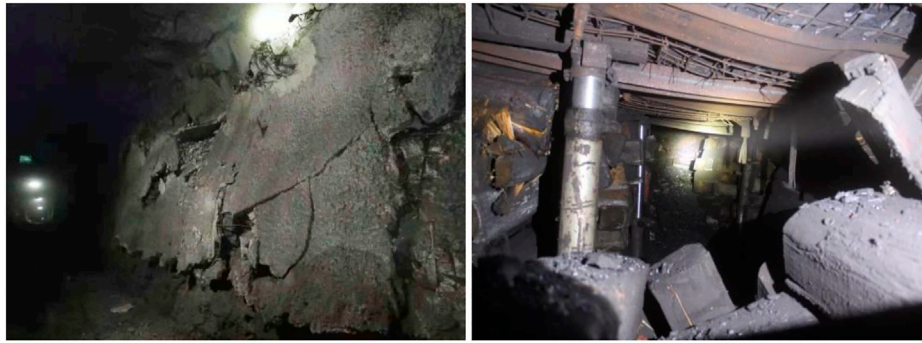
FIGURE 1 Deformation of strong dynamic pressure roadway in the Datong mining area.
