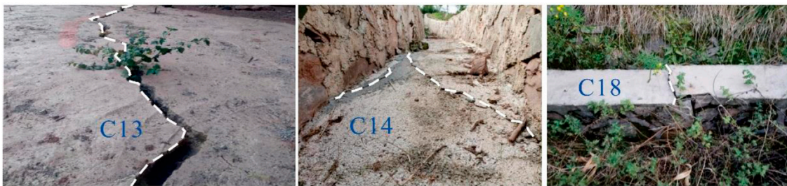
FIGURE 6 The typical old cracks developed in 2007 and 2008 due to deformation of the old Dashuitian landslide.
