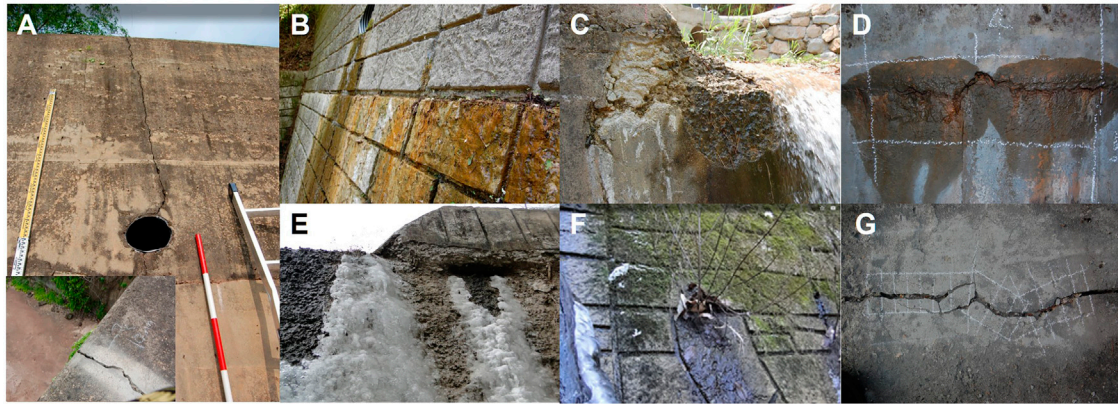
FIGURE 7 | Various deterioration types observed on concrete check dams. (A) vertical through crack and displacement caused by drying shrinkage cracking; (B) water leakage from a gap in a horizontal construction joint; (C) exposed aggregate and spalling, respectively, due to erosion at the spillway; (D) leakage and efflorescence at a horizontal construction joint; scaling and spalling of the downstream face due to freezing and thawing; (E) (F) uncontrolled vegetation around a drainage channel; (G) through crack and dam crest stepping.
