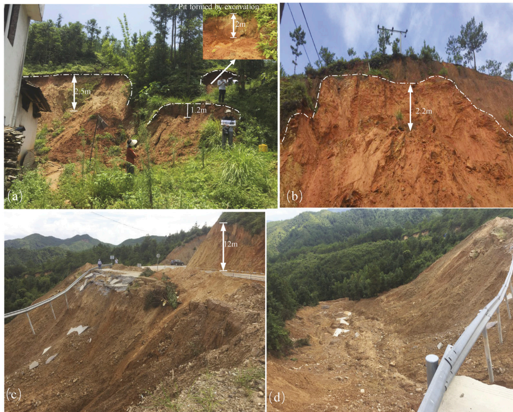
FIGURE 8 | (A) Small-scale collapse landslide on a weathered granite slope behind a house in Qixia Village, Ganzhou City. (B) Collapse landslide on a steep slope on weathered granite, behind the Dinglong Village Committee House, Ganzhou City. (C,D) Steep, high slope on metamorphic rock next to the Kuantian County Road (Ganzhou City), which was damaged by a flow-collapse landslide.
