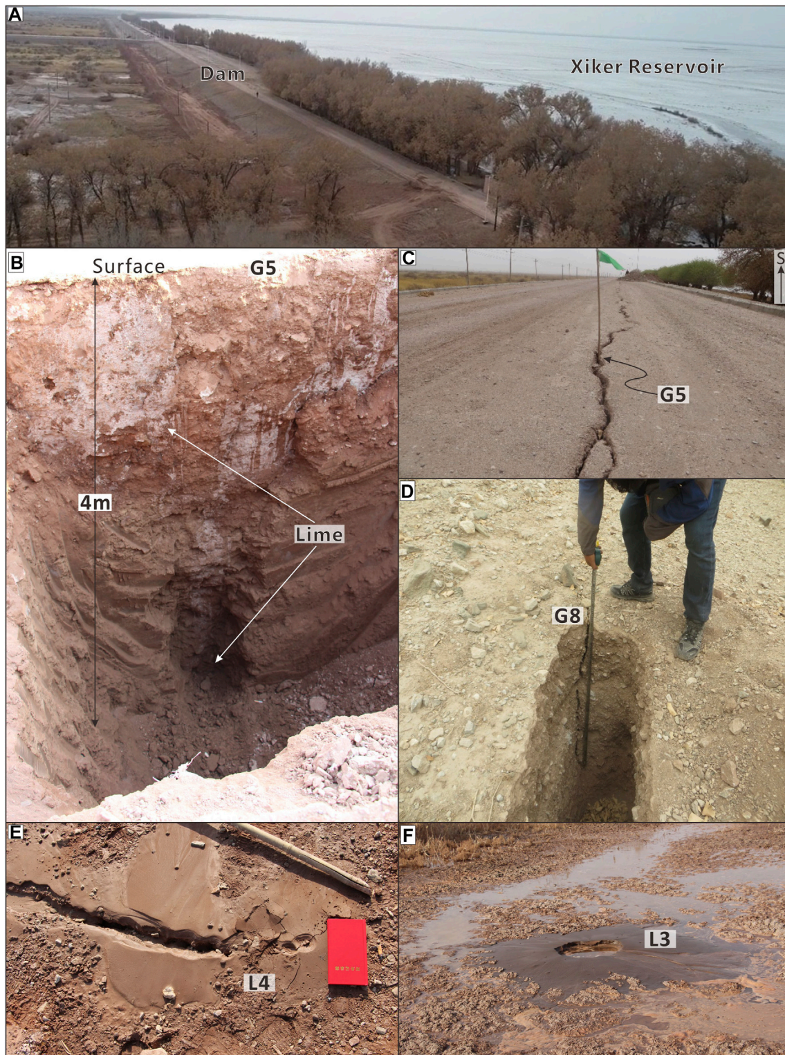
FIGURE 3 | (A) A drone image of the Xiker reservoir and dam (taken on January 20, 2020). (B) A trench dug for the G5 dam fissure. Before excavation, lime was poured along the G5 dam fissure. The maximum depth of G5 was 4 m. (C) G5 is a tensile dam fissure with a staggered distribution. (D) G8 is similar to G5 in that it is the other major fissure in the dam. (E) A recent image of sand liquefaction site L4. The sand volcano is distributed in a beaded pattern. (F) The largest sand volcano at sand liquefaction site L3.
