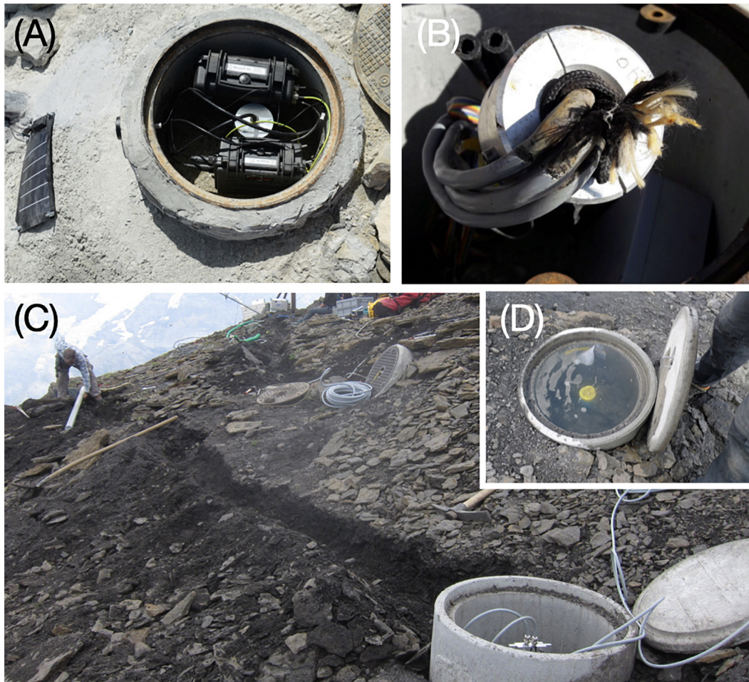
FIGURE 6 | Battery and logging system in a concrete chamber on Wisse Schijen, Switzerland (A, photo: M. Phillips). Damaged cables due to pressure from the lid as a result of subsidence on Murtèl-Corvatsch, Switzerland (B, photo: A. Hasler). Trench and protective casing (white casing in background of the picture) for the cables between the borehole and the instrumentation on Schilthorn, Switzerland (C, photo: A. Hasler). Concrete chamber filled with water above the top of the borehole casing after snow melt on Schilthorn, Switzerland (D, photo: A. Hasler).
