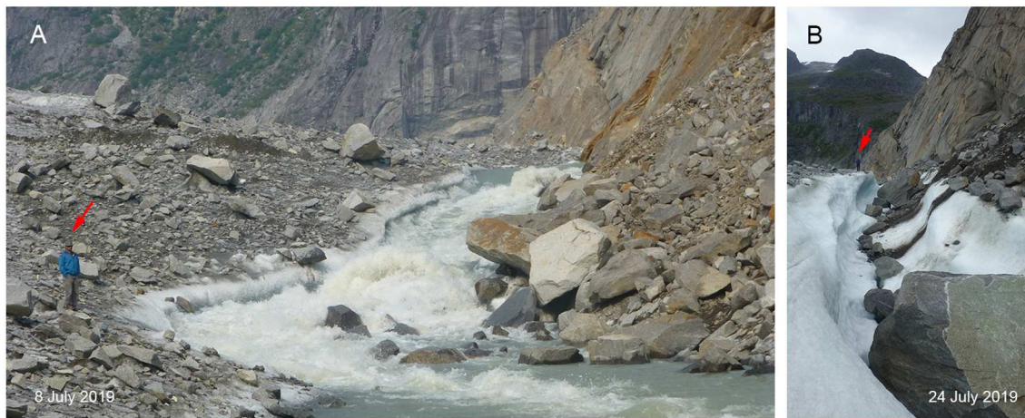
FIGURE 13 | (A) Spillway during the second day of overflow on 8 July 2019. (B) Remnant spillway after 6 days of overflow. Note the person for scale (red arrow). Erosion reached up to 4 m in the imaged portion of the channel. The photo was taken on 24 July 2019, ~12 days after overflow ceased. Boulders and rocks partly filling in the channel originated from the ice-cored moraine.
