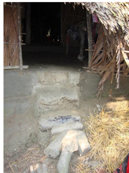
D A local adaptation strategy to fight against sudden storm surges by building clay steps higher than the ground level (Shabajpur village).
