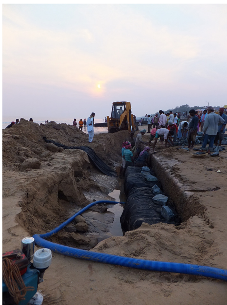
FIGURE 4 Infrastructure project: Embankment construction work in progress along the coastline in Digha. Source: Authors.
