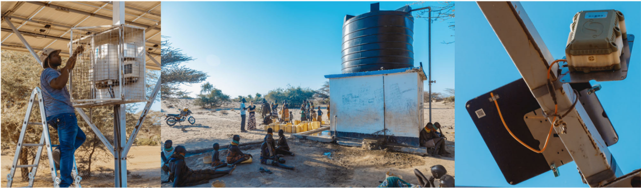
FIGURE 2 | A typical groundwater borehole in Turkana, Kenya (center). Electrical monitoring sensors are installed at the pump controller (left), and wireless transmit data to a self-powered satellite or cellular transmitter ( www.sweetsensors.com ).
