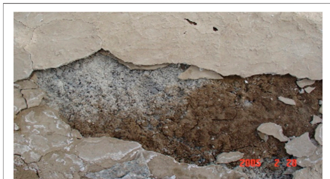
FIGURE 4 | Thaumasite formation under external sulfate attack (groundwater [\text{SO}_4^{2-}] = 653 \text{ mg/L} ) in the Yongan Dan in Keshi of China (Mingyu et al., 2006).
