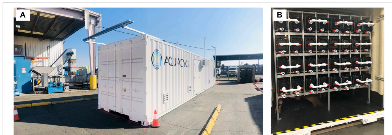
FIGURE 9 | 12-m C-BETT system installed at a soda manufacturer customer site. (A) Outside view of C-BETT and (B) BETT reactors arrangement inside C-BETT.
