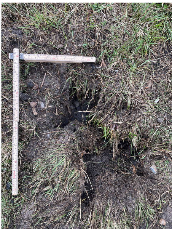
FIGURE 10 Test area B1 with burrow hole after testing.
