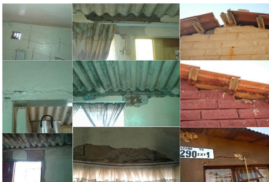
FIGURE 9 Horizontal cracks observed in low-cost URM buildings after the 2014 Orkney earthquake.
