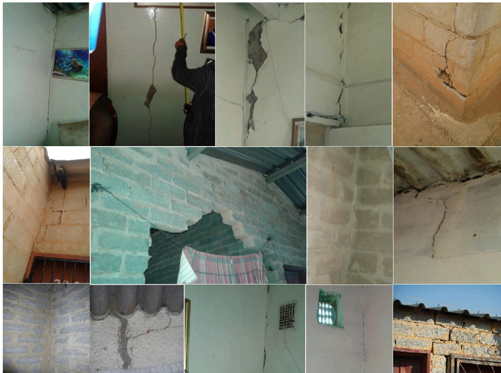
FIGURE 10 Vertical cracks observed in low-cost URM buildings after the 2014 Orkney earthquake.
