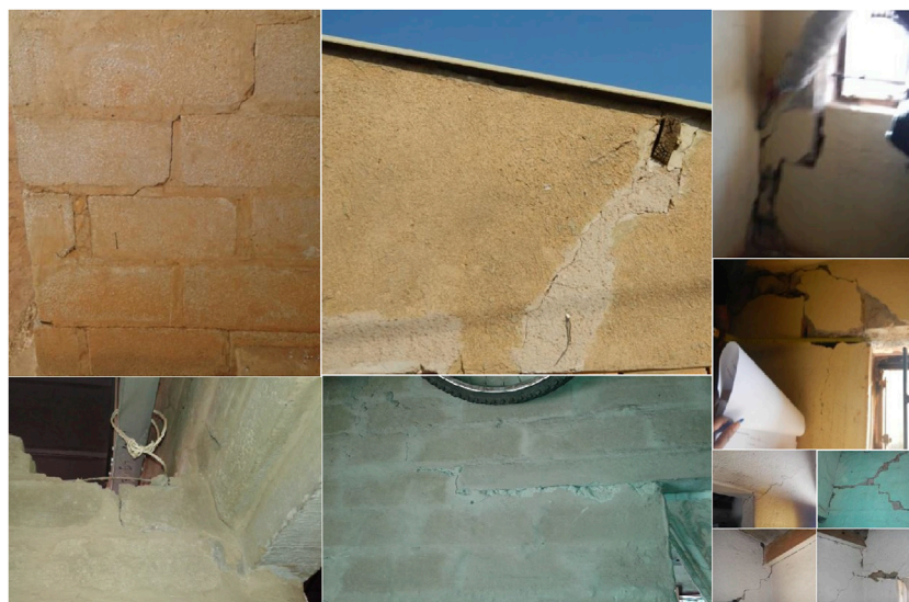
FIGURE 8 Diagonal cracks observed in low-cost URM buildings after the 2014 Orkney earthquake.
