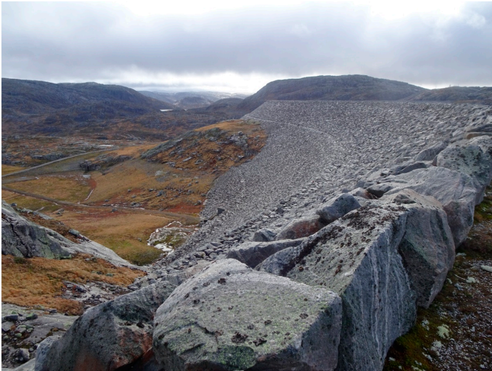
FIGURE 1 Placed riprap on the downstream slope of Storvass dam, Norway. (Image courtesy of the Norwegian University of Science and Technology.)
