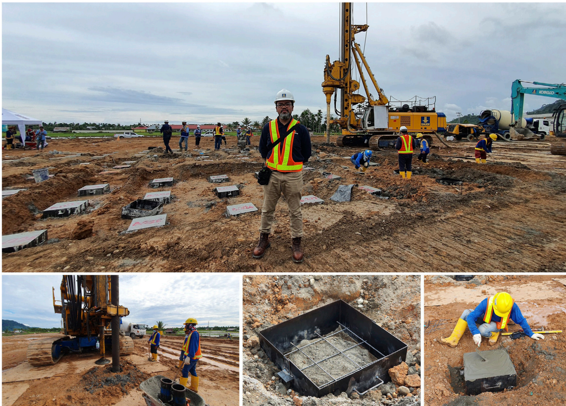
FIGURE 3 Construction of IKM piles in the trial embankment area (source: PT Bauer Pratama Indonesia).
