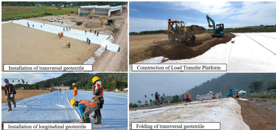
FIGURE 4 Installation of the high-strength geotextile and construction of the LTP in the trial embankment area (source: PT Bauer Pratama Indonesia).
