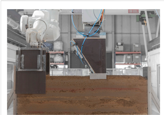
FIGURE 1 Robotic Rammed Earth process at the Institute of Structural Design of Technische Universität Braunschweig (Schweiker et al., 2021).
