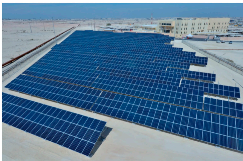
FIGURE 5 Bahrain Oil Company's 1 MW solar polycrystalline solar PV installed on an area of 14900 m 2 at Awali, Kingdom of Bahrain.
